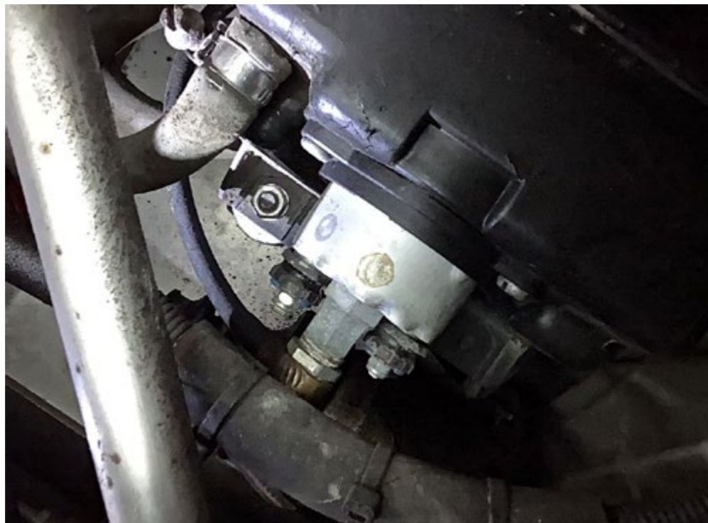
Die damalige Dichtung des Benzinfilters versagte, was fast zur Katastrophe führte. The fuel filter seal used at the time failed, which almost led to disaster.
